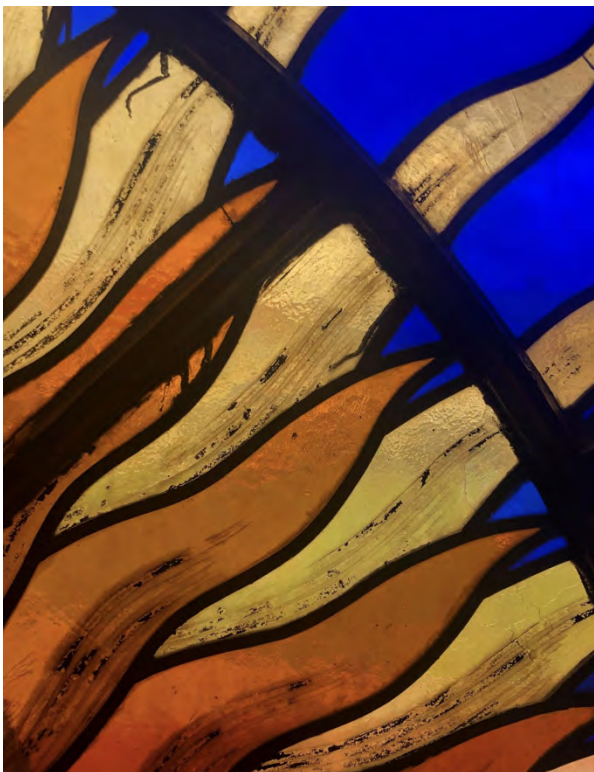
Figure 63. Paint-loss of Callmänder's stained glass in Varberg's church. Photo: Eisfeldt, 2022
