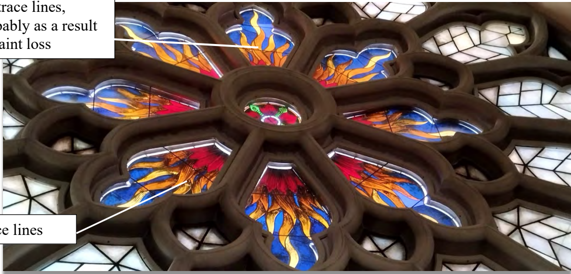
Figure 44. The west rose window of Oscar Fredrik's church. In the photo paint loss is visible, and can be seen especially on the upper side of the window. Photo: Eisfeldt, 2022
