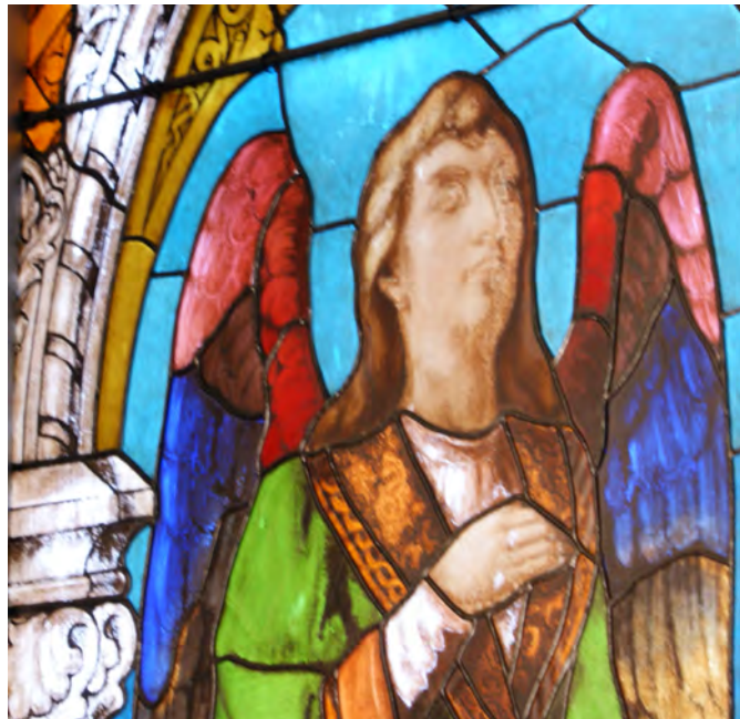
Figure 56. Photo of face with severe paint loss in the left window in the choir of Jonsered church. Photo: Eisfeldt, 2022
