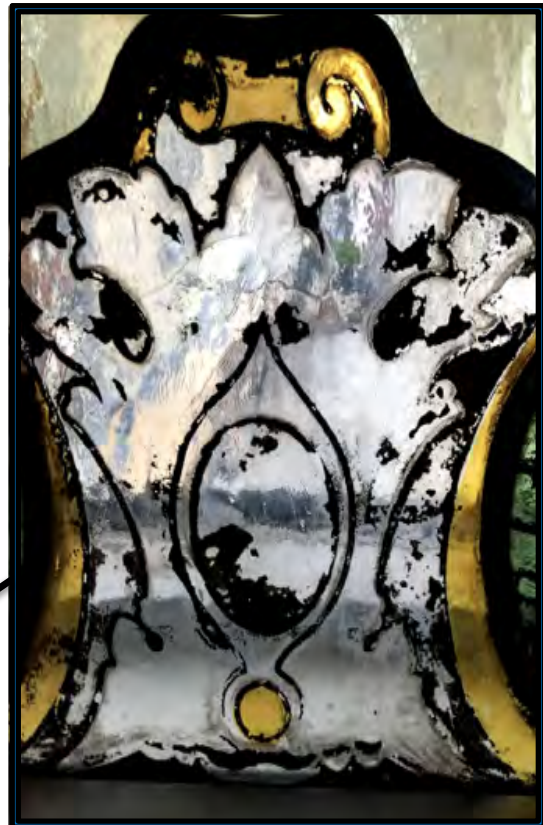
Figure 66. Close-up on the paint loss of the window shown in figure 65. Photo: Eisfeldt, 2022
