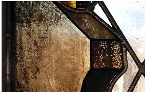
Figure 24. Photo of the window of St, Matheus showing paint loss. Photo: Eisfeldt, 2022
