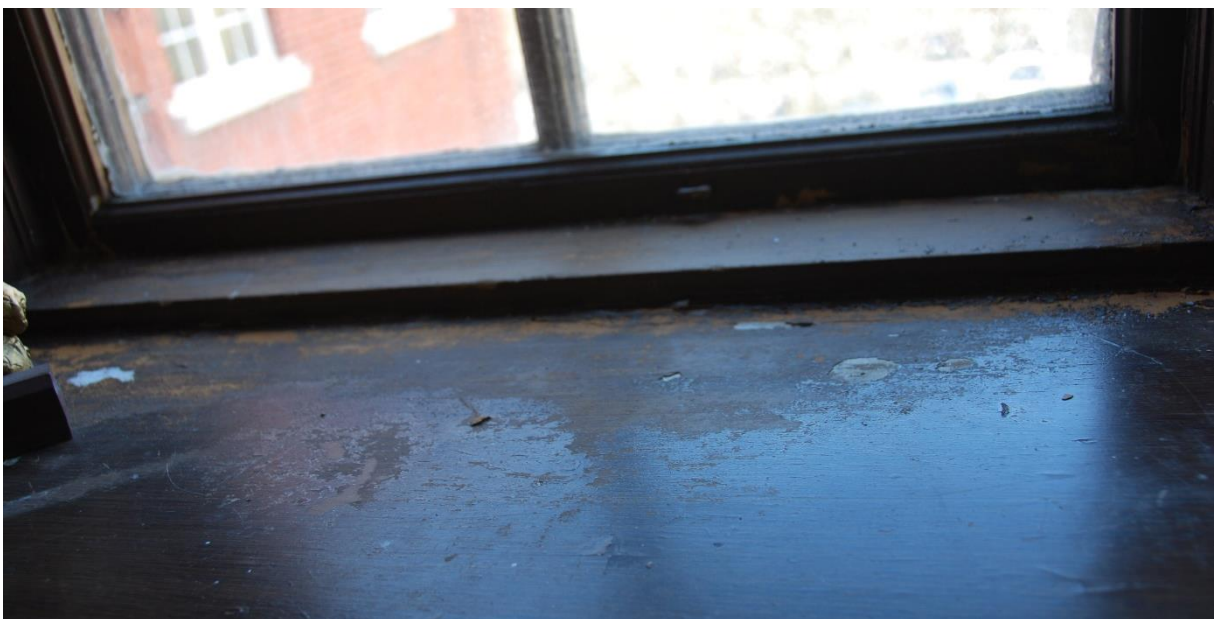
Figure 6. Flaking paint on interior window sill.
