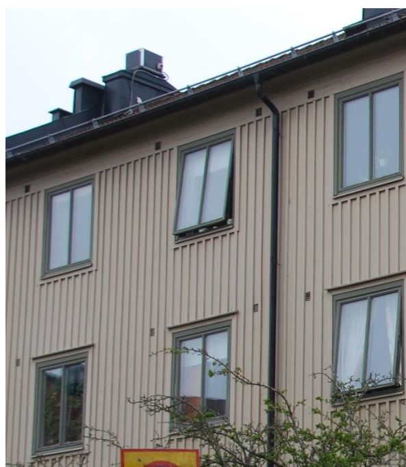
Figure 18. When open, the inappropriate window type is exposed.
