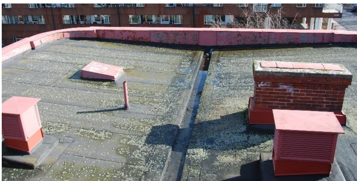
Figure 8. Stagnant water in roof valleys and roofing felt covered in lichen.
