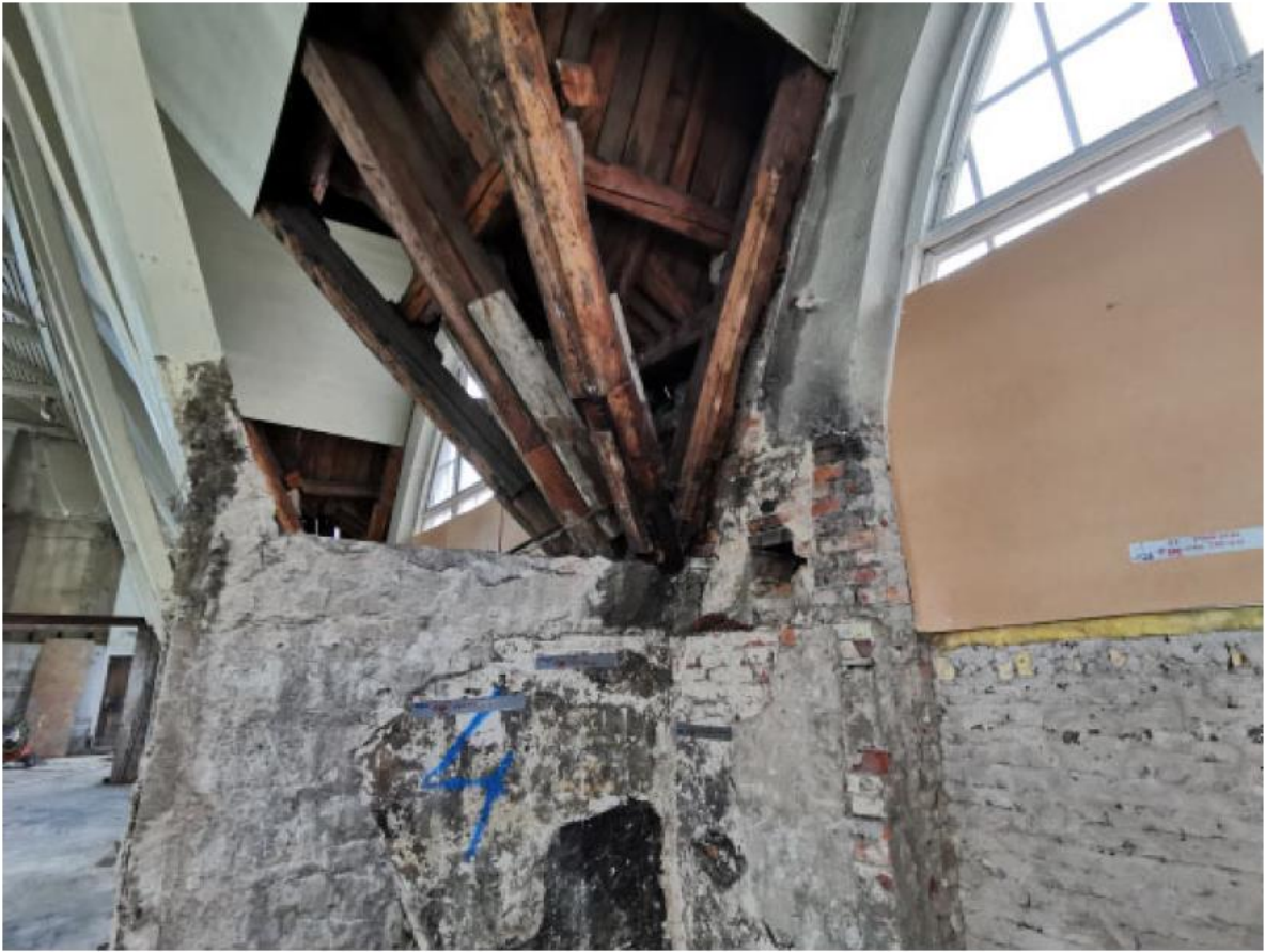
Figure 32. Damage to the roof truss in the connection points to the counterforts, especially near the exterior wall. By Mattson, 2022.
