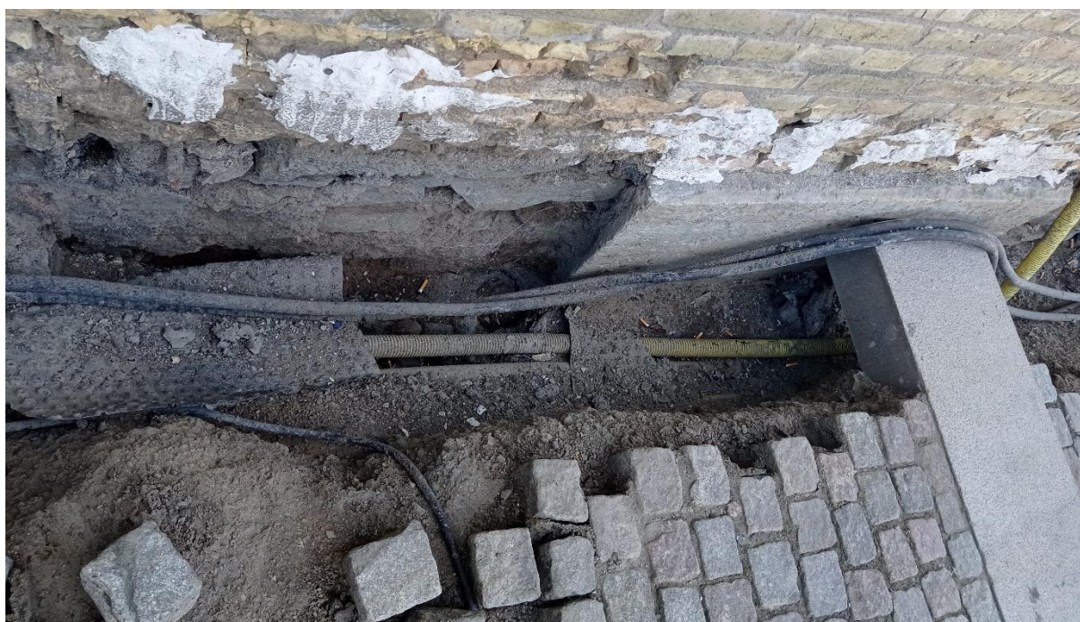
Figure 31. The lime stone base is partially submerged under-ground due to elevation of the ground level.
