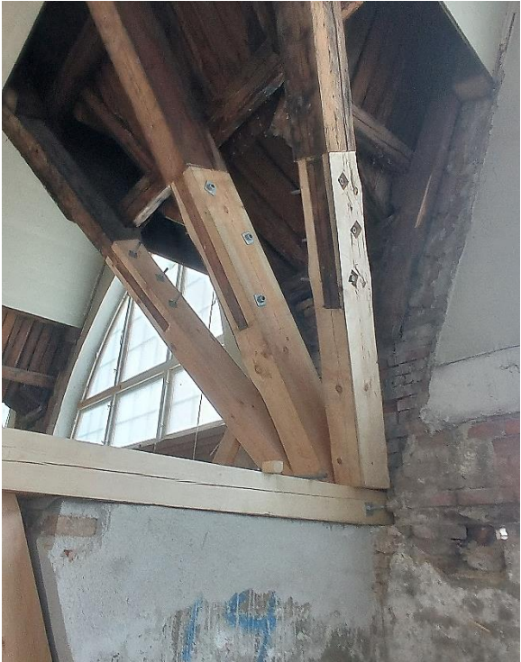
Figure 28. Repair on hidden part of structure.
