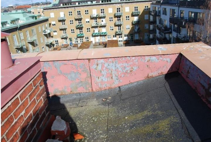
Figure 9. Flaking paint on metal roofing covering balustrade.
