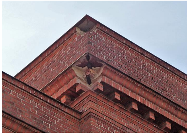
Figure 4. Damaged corner of the dentils frieze.
