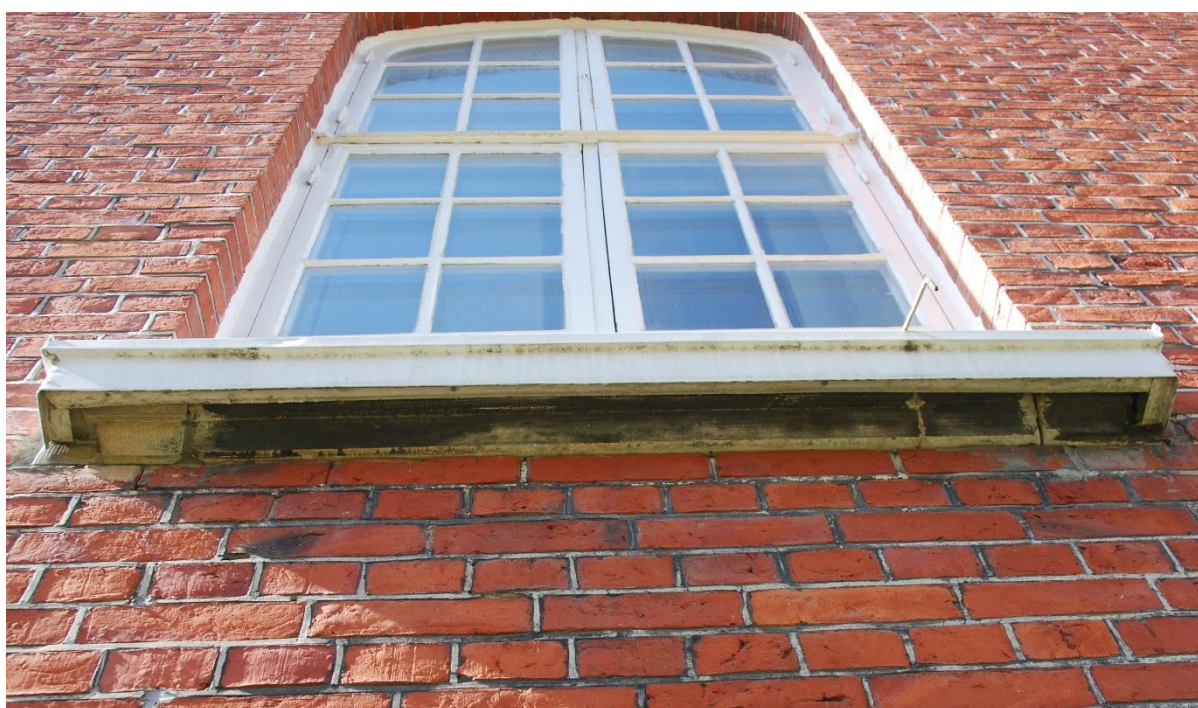
Figure 7. Exterior window sills blackened underneath.
