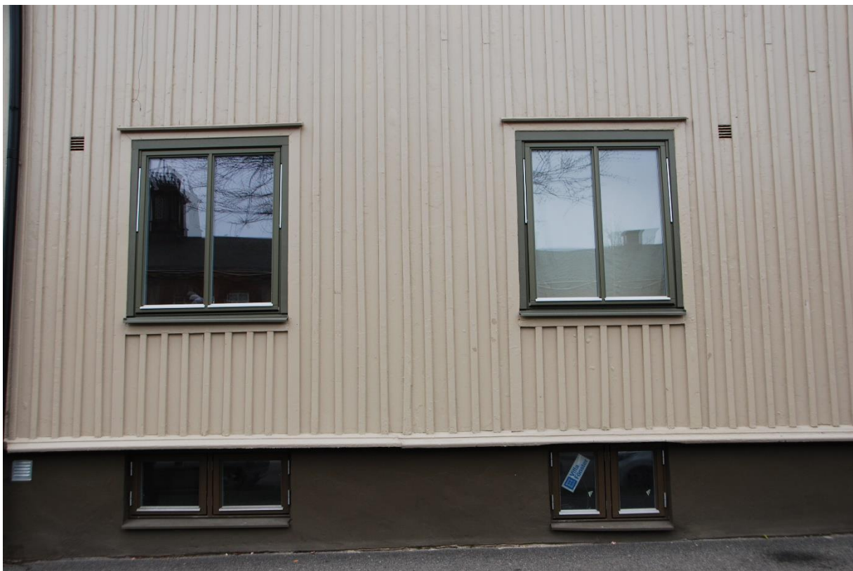
Figure 14. Appearance of the street façades; connection between concrete base and upper wood construction.
