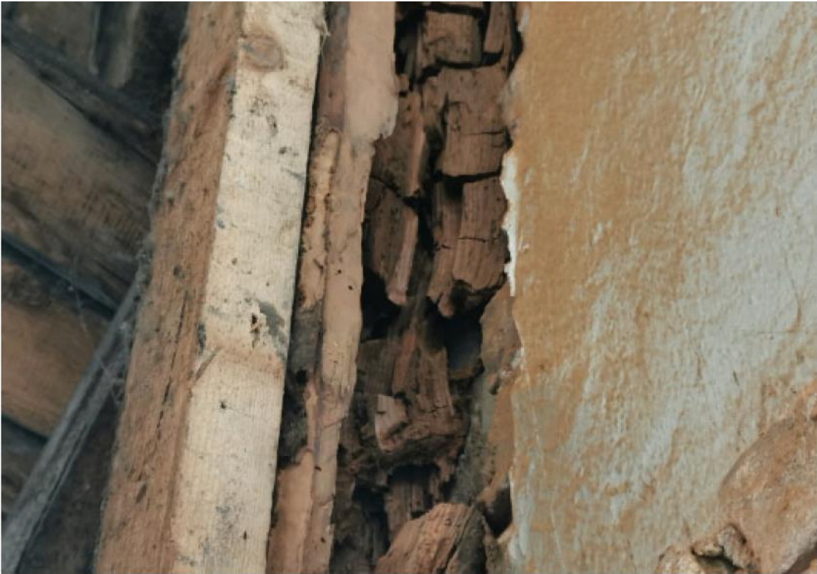
Figure 33. Close-up of the damage in one of the connection points. By Mattson, 2022.
