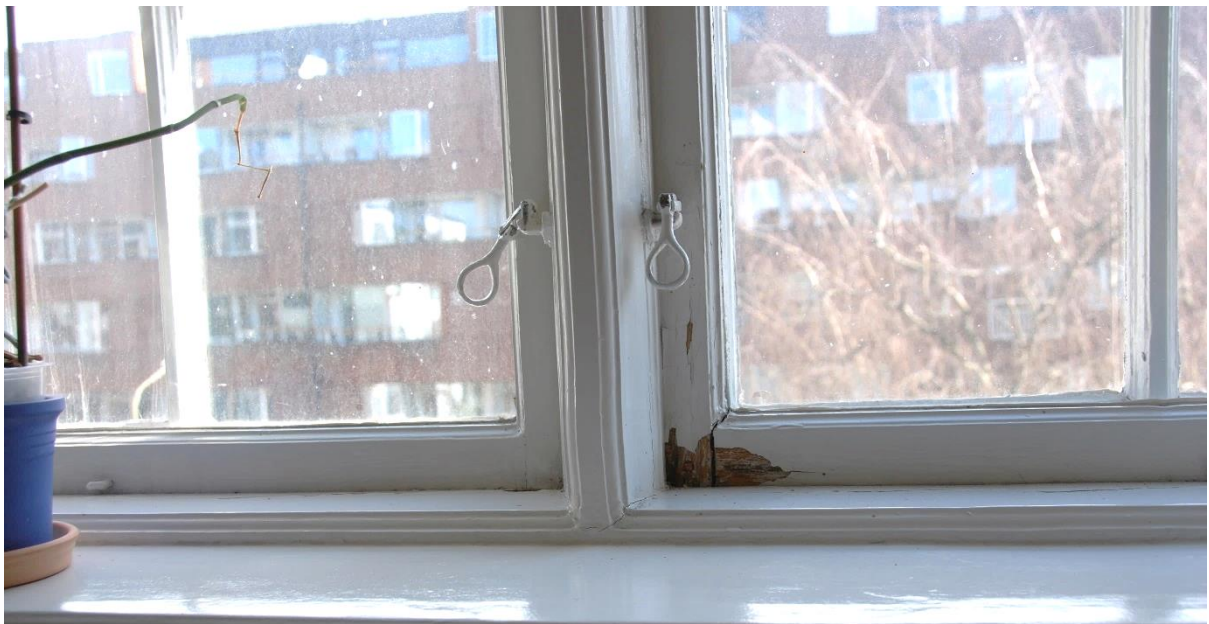
Figure 5. Flaking paint and potentially damaged wood in lower corner of window sash.
