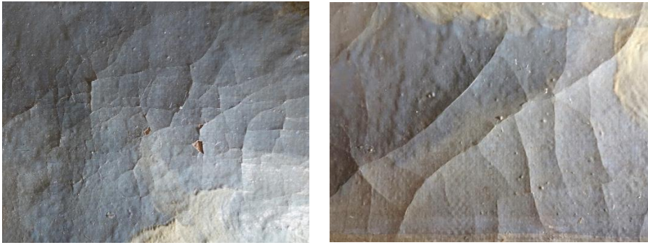
Figure 4: Close-up of delaminating, cracking and flaking paint. Figure 5: Close-up of cupping paint.
