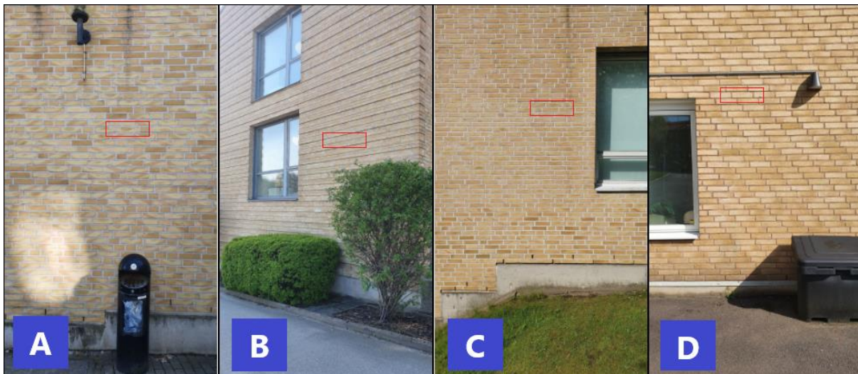
Figure 2. Pictures showing the four sides of GVC where A is the North East side, B the South East side, C the South West side, and D the North West side, with the respective points on the wall marked with red where the measurements were taken.
