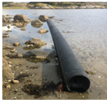
Old sewage pipe
