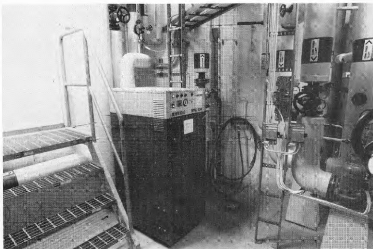
Figur 7.1 Elpanna i undercentral
