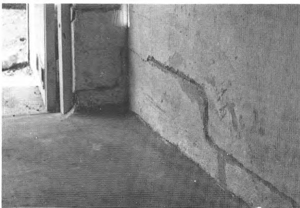
FIG. 7. Spricka i väggen mellan garage och hobbyrum. Crack in wall between garage and hobby room.
