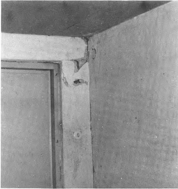
FIG. 5. Spricka i garageportomfattning. Crack in garage doorway.
