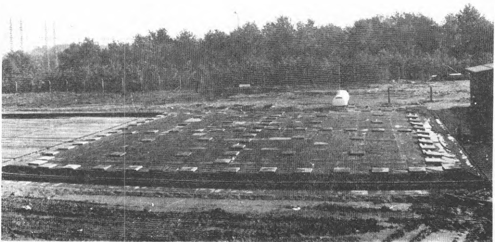
Fig. 3. The final plant. The "dry dock" where construction of the lid was undertaken, is partly seen to the left.
