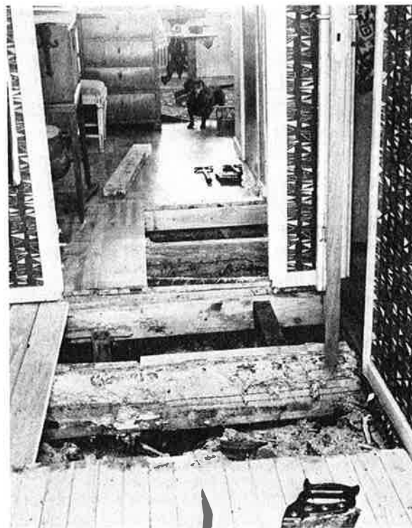
Ovan: Fig. 6. Flera intressanta skador har undersökts av institutet i samband med skadeinventeringen. Bilden visar rötskadat träbjälklag i hus utan källare Above: Fig. 6. Several interesting cases of damage have been investigated by the institute in connection with the schedule of damage. The photograph shows timber joists damaged by rot in a house without basement
